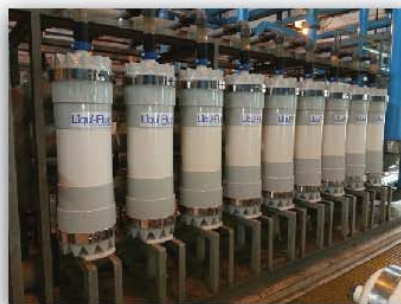
Pre-treatment to Reverse Osmosis
